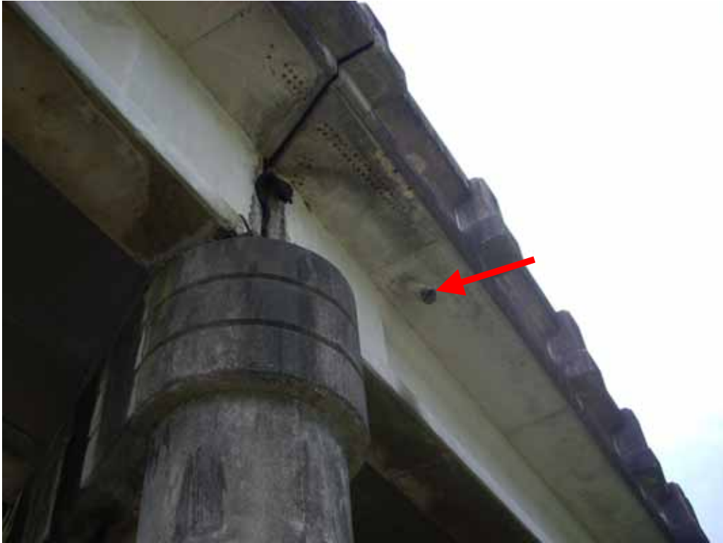
Photograph 3 – Typical view of asbestos containing transite drain pipe located in the bridge deck.
