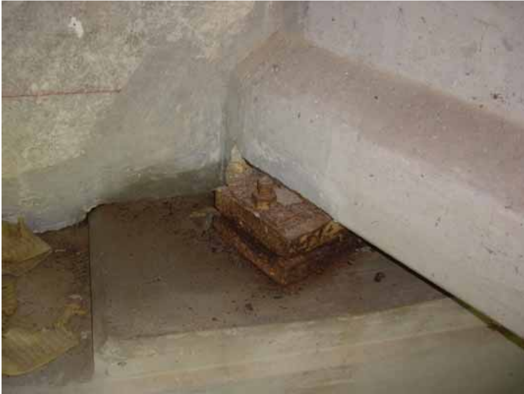
Photograph 5 – Typical view of metal bridge shoe and associated bolt. These components are coated with lead based paint.
