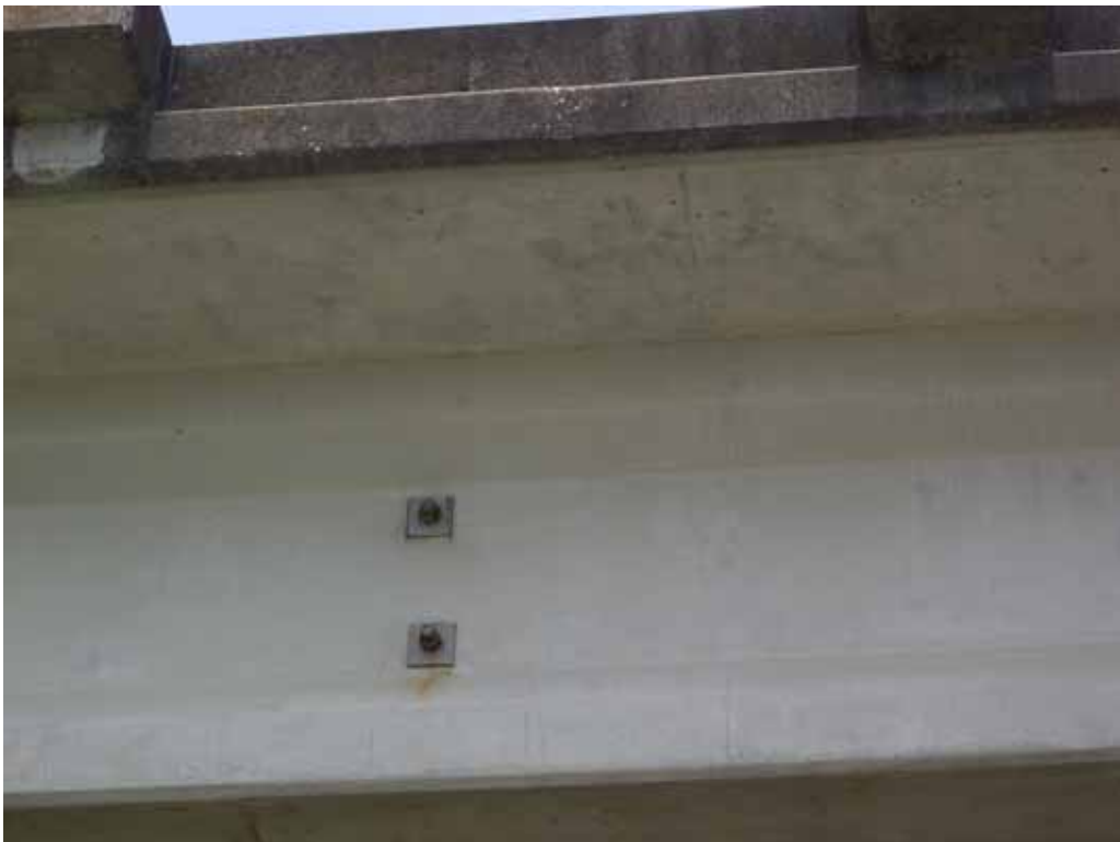
Photograph 4 – Typical view of steel tie rods and plates located on the bridge structure. These components are coated with lead based paint.
