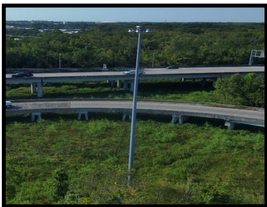
PHOTOGRAPH 3-23: HIGH MAST LIGHT POLE
