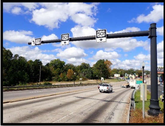
PHOTOGRAPH 3-19: MAST ARM (FRONT)
