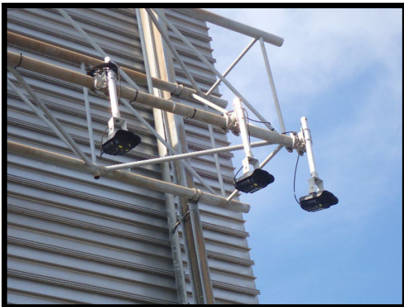
PHOTOGRAPH 4-19: CAMERAS ATTACHED TO TRUSS
