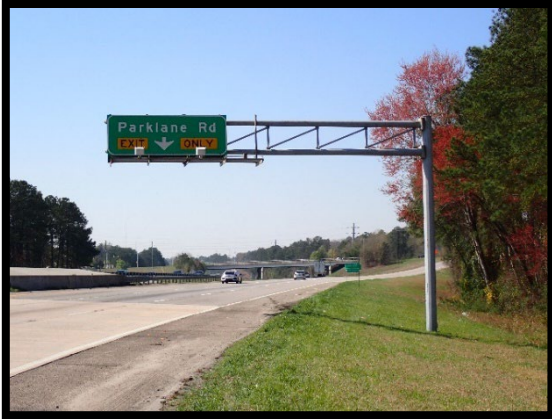
PHOTOGRAPH 3-01: 2-CHORD MAST ARM (FRONT)
