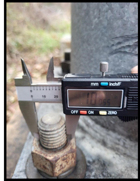
PHOTOGRAPH 3-37: ANCHOR ROD MEASUREMENT WITH CALIPERS
