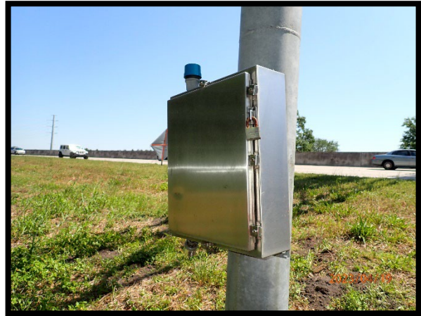
PHOTOGRAPH 4-18: ELECTRIC BOX ATTACHED TO COLUMN
