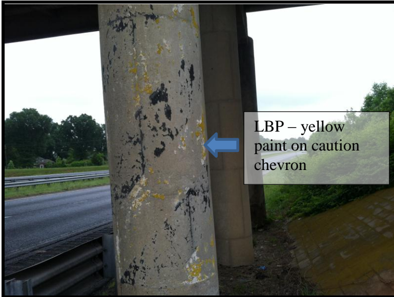
5 Lead sample from caution chevron on piers.
