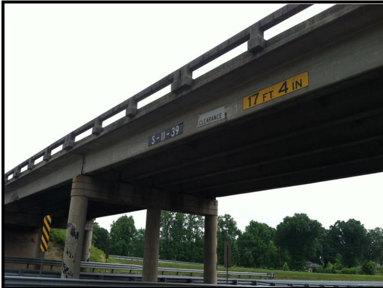
1 Bridge S-11-39 on Green River and Macedonia road over I-85 General view from I-85
