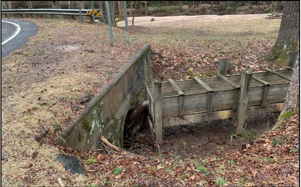
Figure 37. View of Pipe in Culvert Emptying Into Rebuilt Flume within the Original Mill Race, Facing South.
