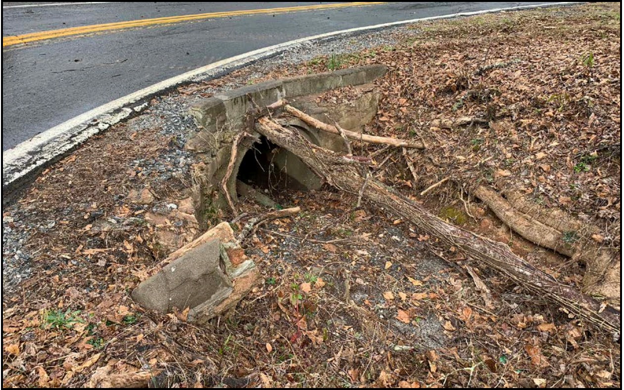
Figure 36. View of Pipe Entering Culvert through Mill Race Passing Under Timms Mill Road, Facing Northwest.
