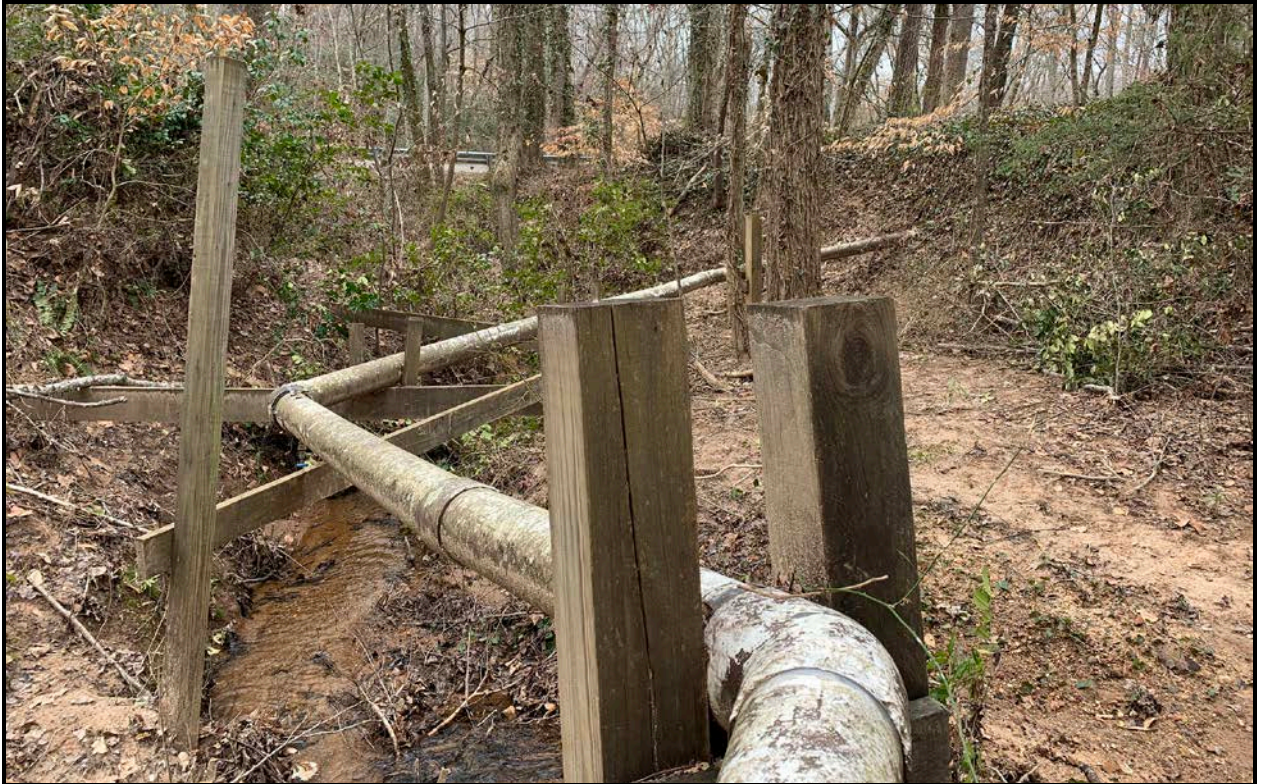
Figure 35. View of PVC Waterpipe Showing Where Pipe Breaches the Mill Race, Facing Southwest.
