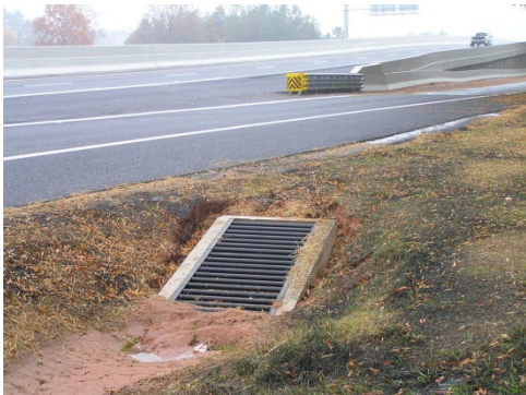
Use Pipe End Structure (719-615-00) when specified in the plans or special provisions. Use pipe end structure in locations where pipe exposed end faces the direction of traffic. Pipe end structures may be used in other locations if approved by the RCE.
