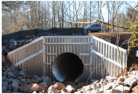
Use Pipe Wingwall
