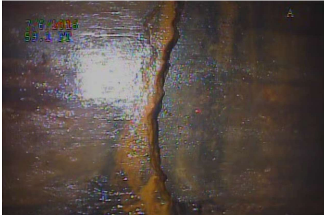
59.1' - CRACK > 12" - LT. SIDEWALL
