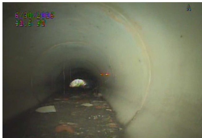
DEBRIS NEAR PIPE OUTLET
