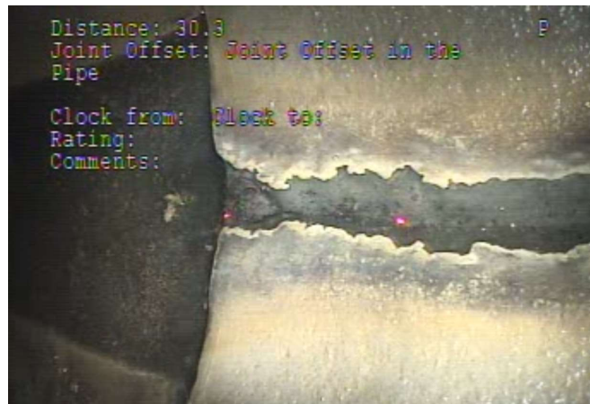
30.3' - JOINT OFFSET IN THE PIPE
