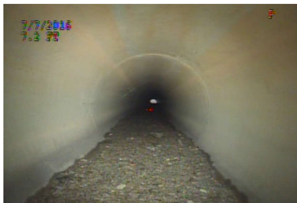
Debris in pipe
