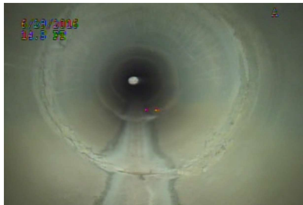
15' - Intruding Sealing Grout
