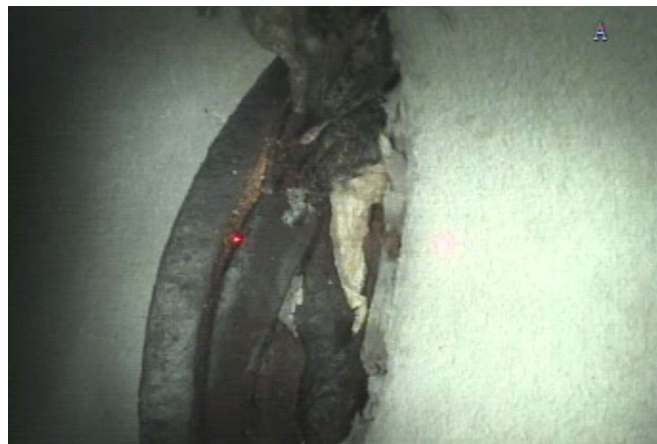
67.8' - JOINT GASKET EXPOSED
