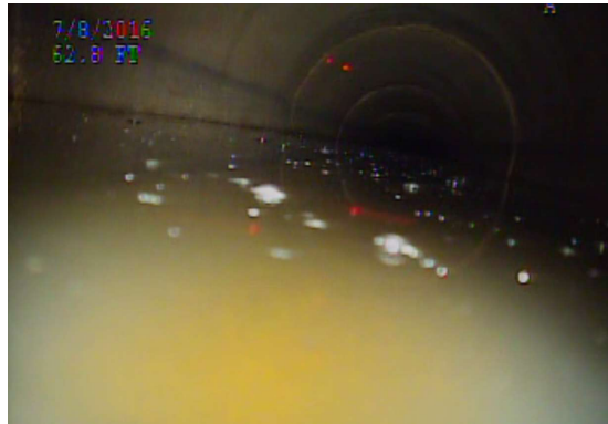
Water in pipe
