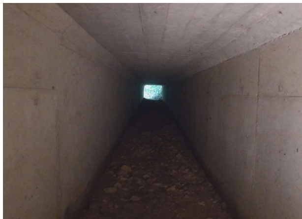
DEBRIS NEAR DOWNSTREAM END
