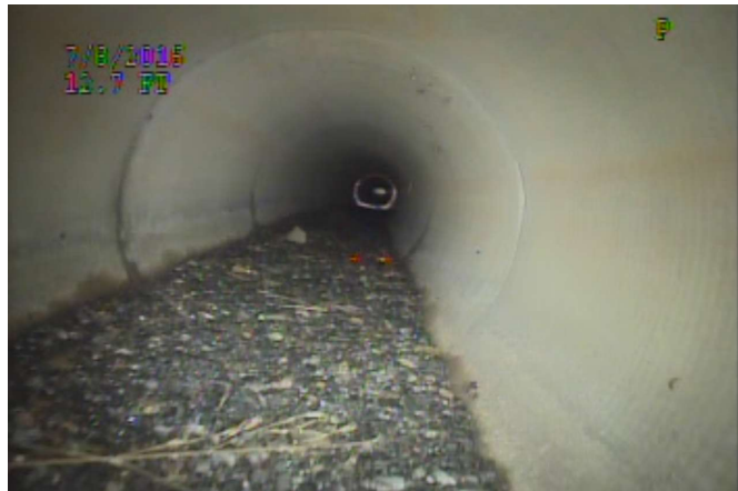
GENERAL - DEBRIS THROUGHOUT
