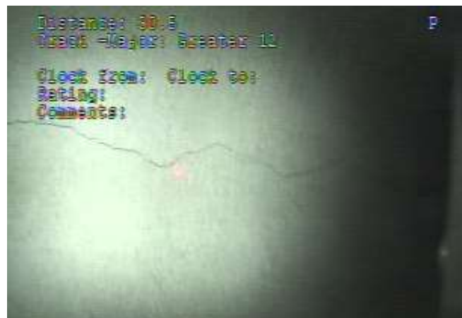
CRACK >12" AT 30.5' (TOP)
