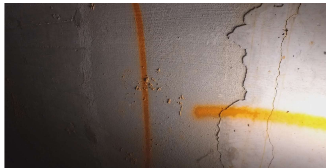
59' - CRACK (RT. WALL - TOP - LT. WALL)
