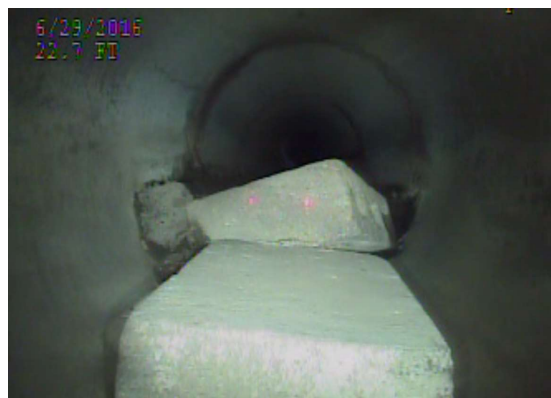
Debris in pipe
