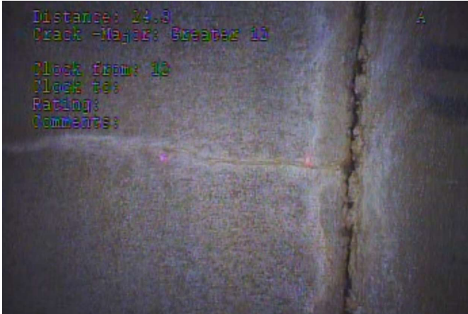
24.8' - CRACK > 12" (ENTIRE LENGTH OF PIPE)
