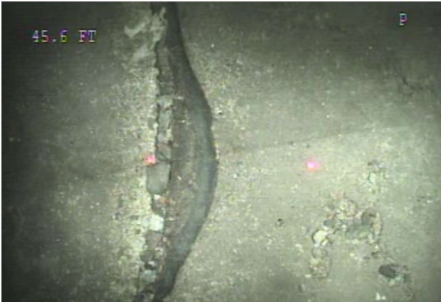
45.6' - JOINT GASKET EXPOSED
