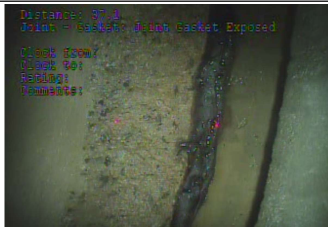
37' - JOINT GASKET EXPOSED
