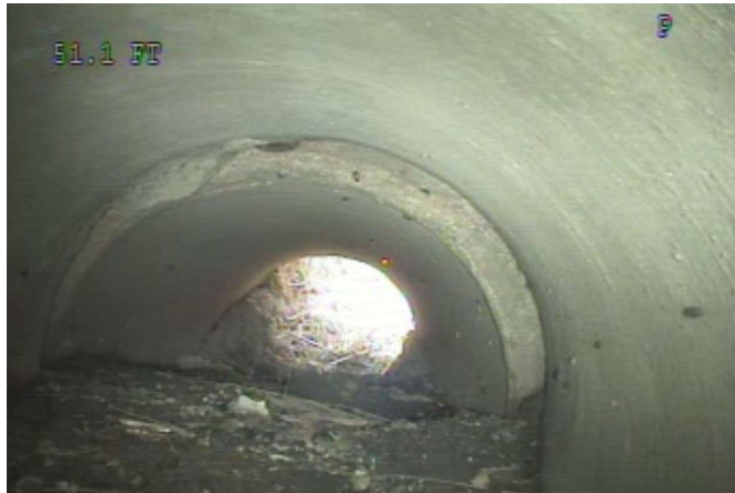
51.1' - JOINT SEPARATED > 1"; DEBRIS
