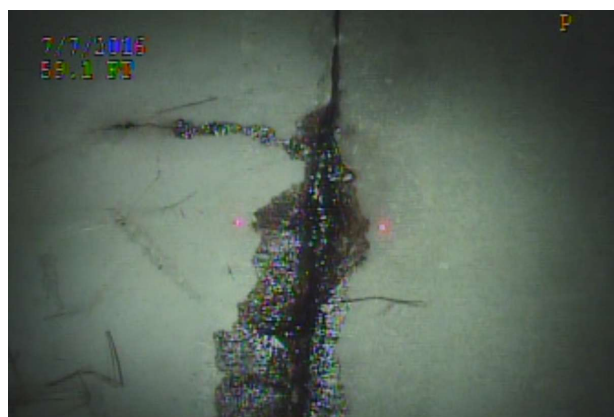
59' - Infiltration in pipe
