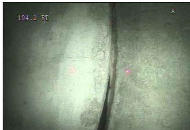
Misaligned Joint at 104.2'
