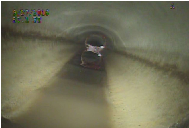
DEBRIS AT DS END CAUSING PONDING IN PIPE
