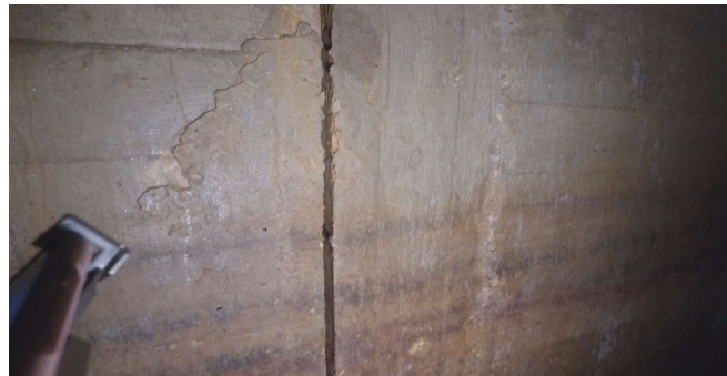
108' - WIDE DISPLACED SEAM (LT.)
