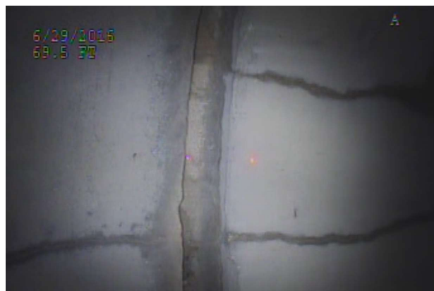
70' - Joint Separated > 1"/Multidirectional Crack
