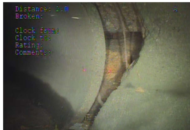
2' - Broken pipe at joint
