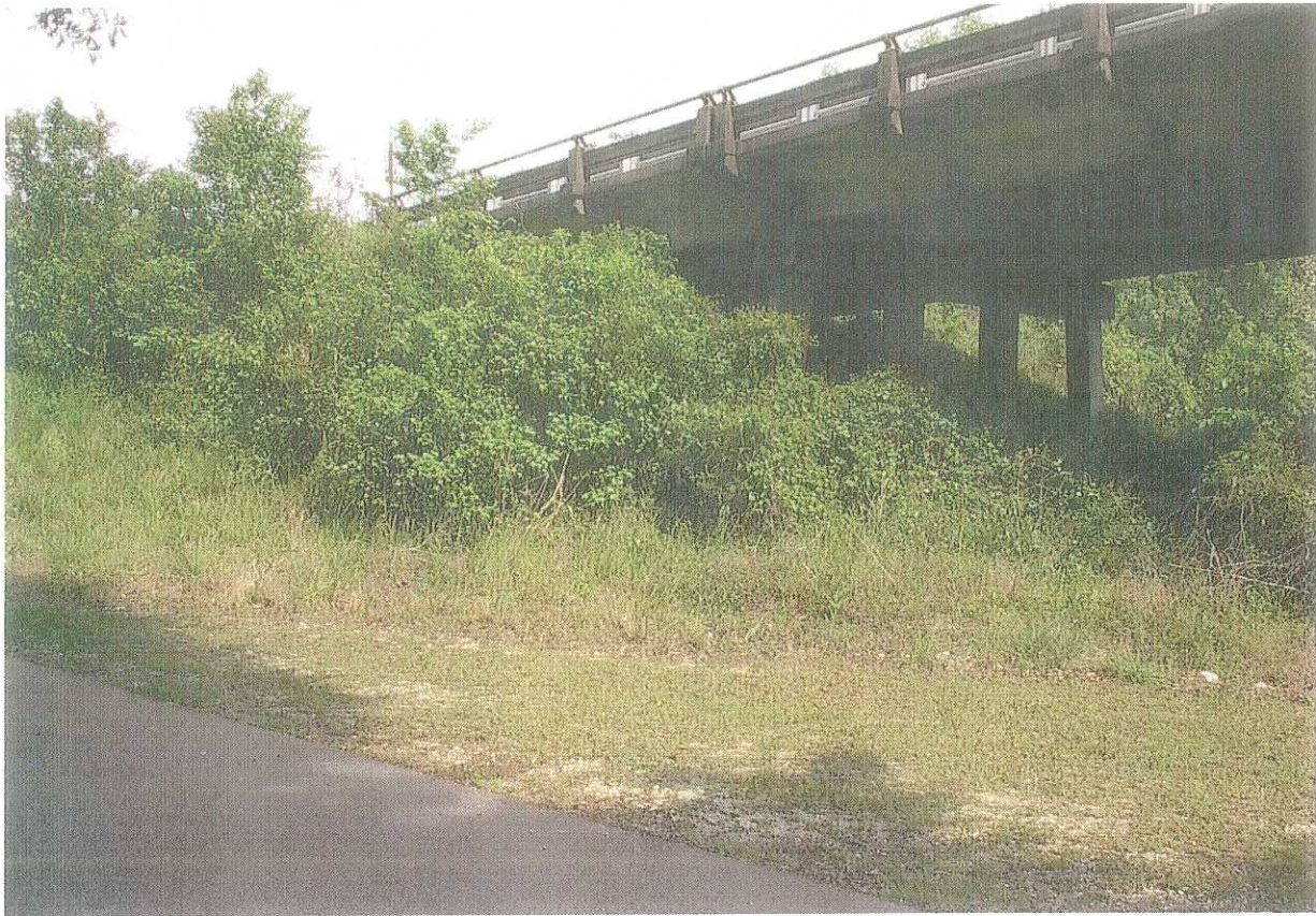
PLATE 4 - View of north abutment of the Pee Dee River bridge from the marina access road. Boring B-4 is located nearby. Height of embankment at abutment is approximately 20 feet.
