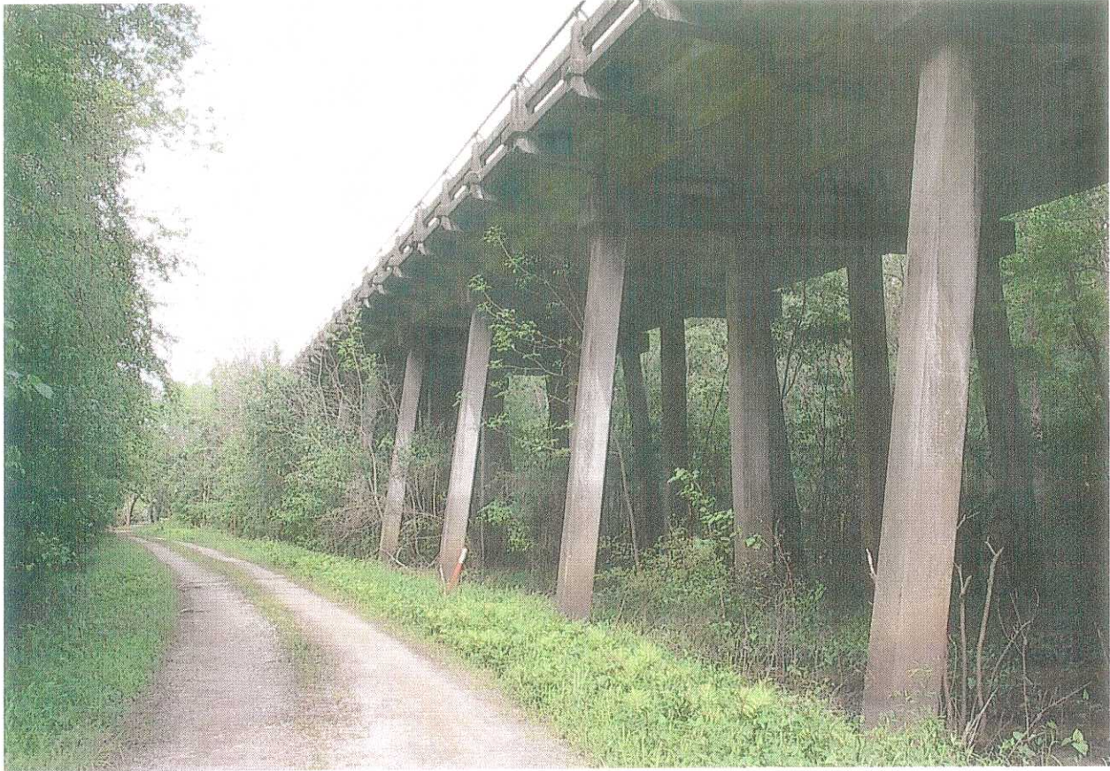
PLATE 9 - View of approach bents on south side of main PeeDee River Bridge. Bents are supported by 18-in square precast piles which bear in non-liquefiable soils on this side of the river.
