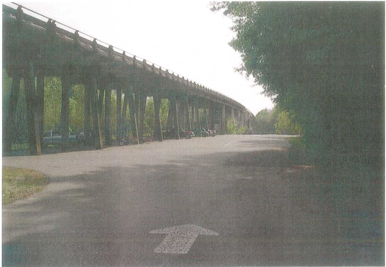
PLATE 5 - View of PeeDee River Bridge looking south from entrance to marina on north bank. Approach spans are pile bents supported by 18-inch precast concrete piles which extend about 30 feet below the surface and terminate in a zone of liquefiable sands which underlie the alignment north of the river.
