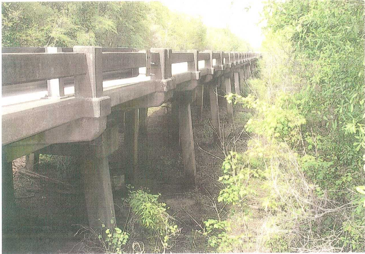
PLATE 2 - View of existing PeeDee Overflow Bridge from near south abutment. At time of visit area beneath bridge structure was almost entirely dry.
