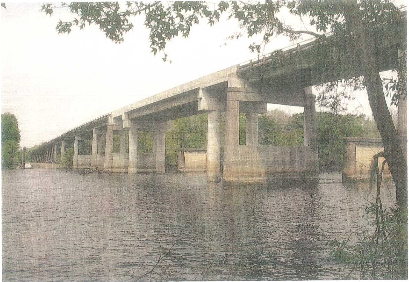
PLATE 1 - View of existing PeeDee River Bridge (Bridge 2) from upstream. Bridge is supported by cast-in-place concrete piers extending below the scour line, in turn supported on timber piles extending approx. 15-30 ft below the base of the piers. The central span was constructed in about 1996 and is supported by drilled shafts bearing in Pee Dee Formation at a depth of about 40-50 feet below the mudline. Piers in river channel beyond the existing bridge were part of old structure that was demolished when the current bridge was built in 1952.
