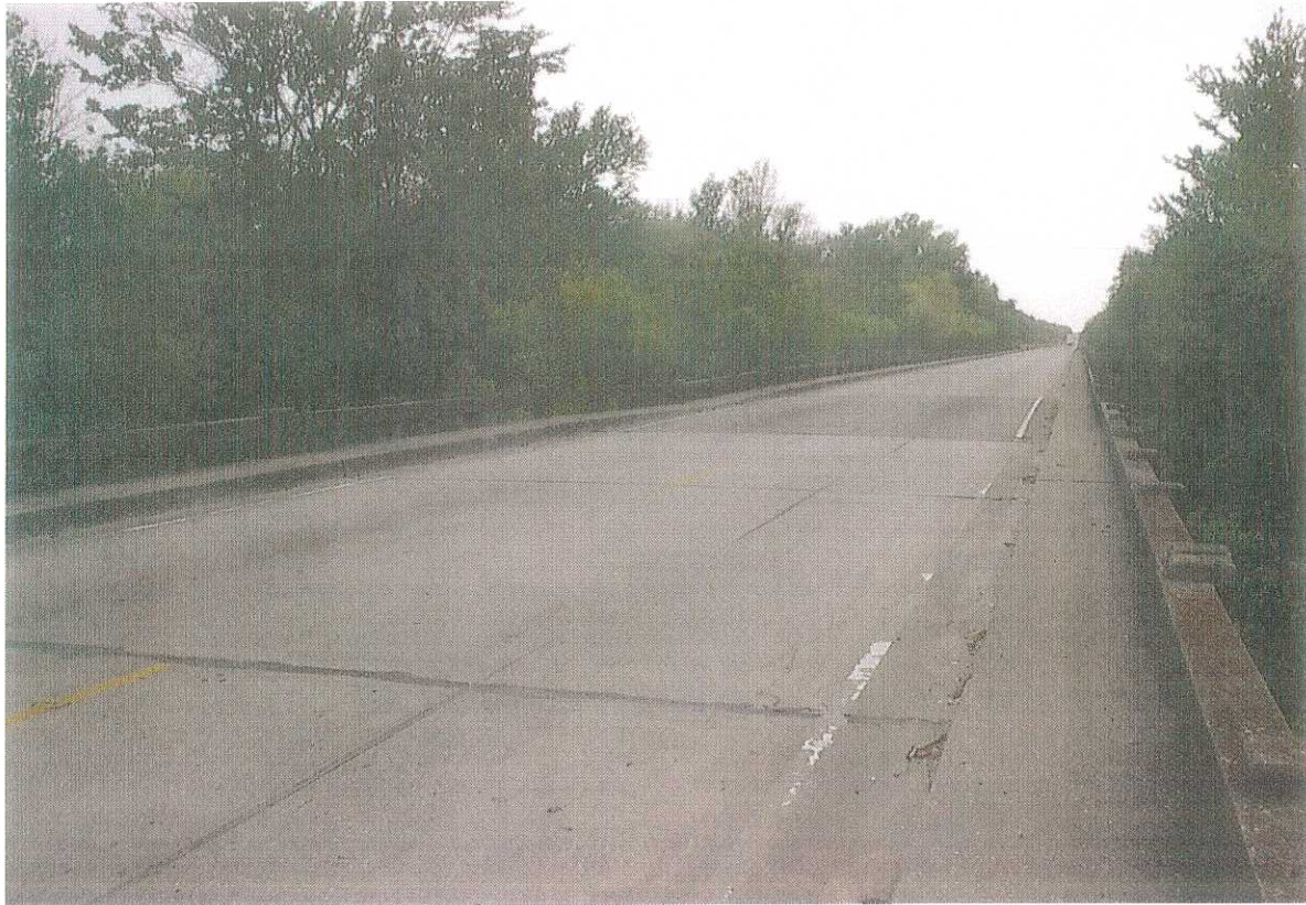
PLATE 3 - View of sag in bridge deck looking south on PeeDee Overflow bridge.
