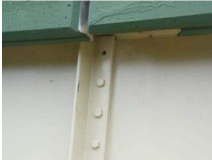
(1020 – Connections) Condition State 2
