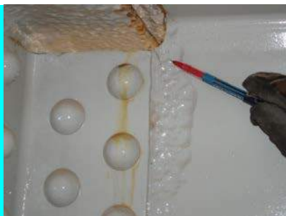
(1010 – Cracking) Condition State 3
