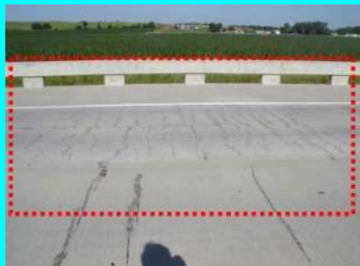
(1130 – Cracking/RC and Other) Condition State 2
