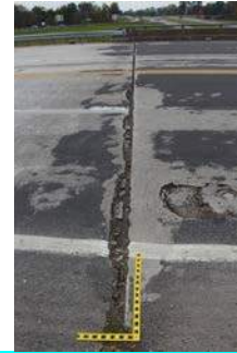
(2350 – Debris Impaction) Condition State 4
