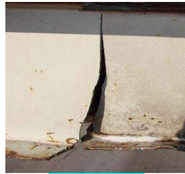
(1010 – Cracking) Condition State 4
