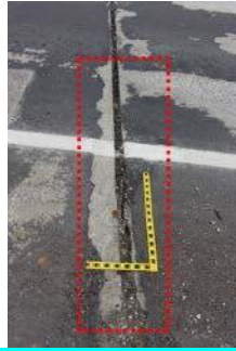
(2350 – Debris Impaction) Condition State 3
