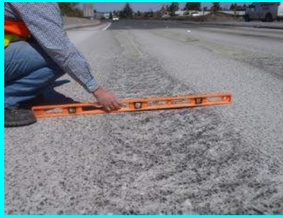
(1190 – Abrasion/Wear) Condition State 3
