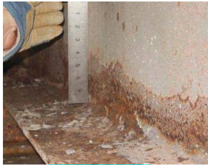
(1000 – Corrosion) Condition State 3
