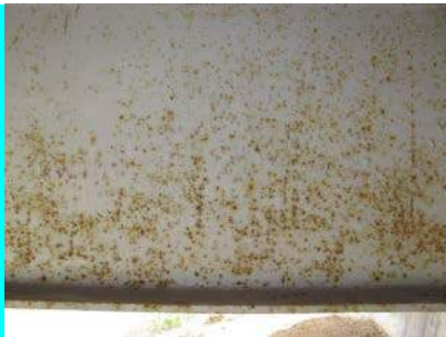
(1000 – Corrosion) Condition State 2
