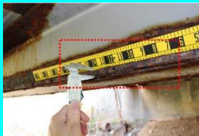
(1000 – Corrosion) Condition State 3
