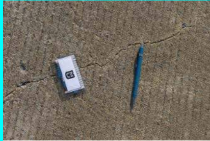
(1130 – Cracking/RC and Other) Condition State 2
