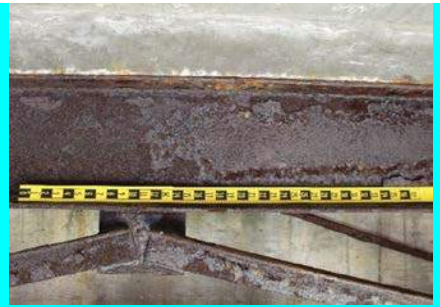
(3430 – Oxide Film Degradation) Condition State 3
