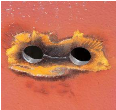
(1010 – Cracking) Condition State 2
