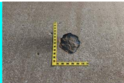
(1080 – Delamination/Spall/Patched Area) Condition State 3
