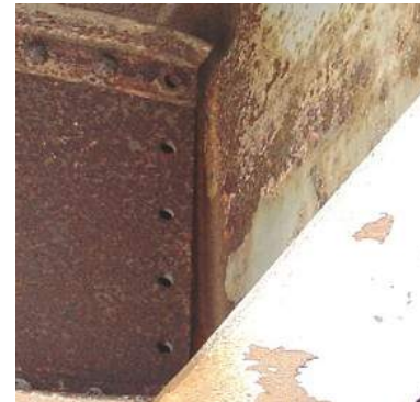
(1020 – Connections) Condition State 4
