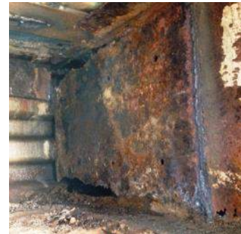
(1000 – Corrosion) Condition State 4
