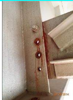
(1020 – Connections) Condition State 3
