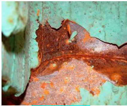
(1010 – Cracking) Condition State 3
