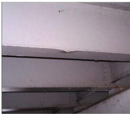
Condition State 2 (Damage)
