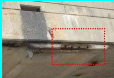
(1090 – Exposed Rebar) Condition State 3
