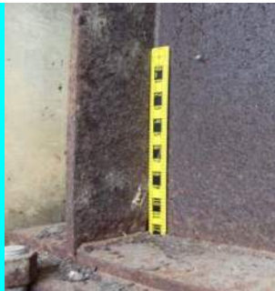
(3430 – Oxide Film Degradation) Condition State 3
