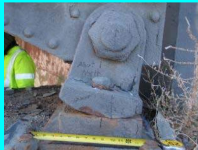
(2220 – Alignment) Condition State 2
