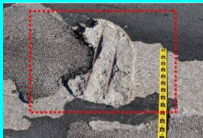
(1090 – Exposed Rebar) Condition State 2
