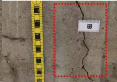
(1130 – Cracking/RC and Other) Condition State 3
