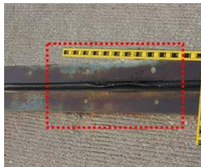
(2330 – Seal Damage) Condition State 3
