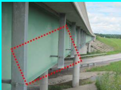
(3410 – Chalking) Condition State 2
