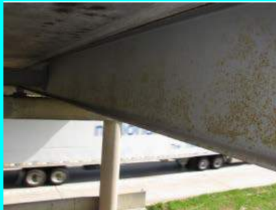
(3440 – Effectiveness) Condition State 2
