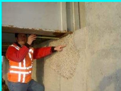
(2240 – Loss of Bearing Area) Condition State 2
