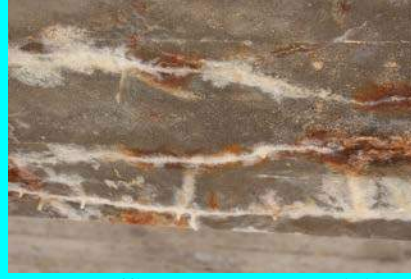
(1120 – Efflorescence/Rust Staining) Condition State 3
