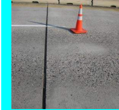
(1190 – Abrasion/Wear) Condition State 2
