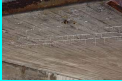
(1120 – Efflorescence/Rust Staining) Condition State 2
