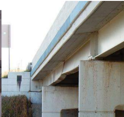
Condition State 3 (Damage)
