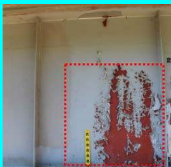
(3420 – Peeling/Bubbling/Cracking) Condition State 2
