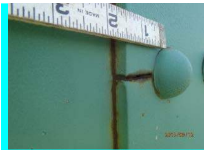
(1010 – Cracking) Condition State 2
