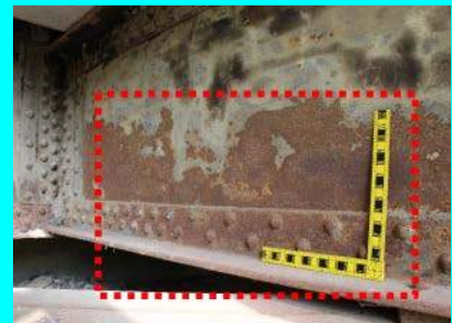
(3440 – Effectiveness) Condition State 4
