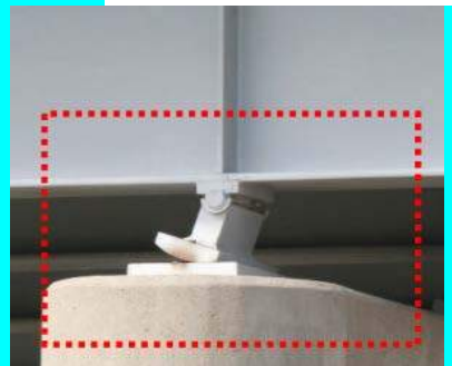
(2220 – Alignment) Condition State 3
