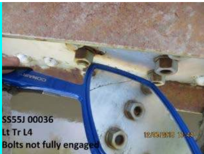
(1020 – Connections) Condition State 2
