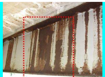
(3420 – Peeling/Bubbling/Cracking) Condition State 4
