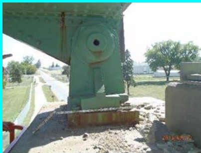
(2220 – Alignment) Condition State 1
