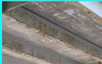
(3440 – Effectiveness) Condition State 3
