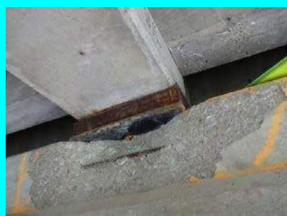
(2240 – Loss of Bearing Area) Condition State 3
