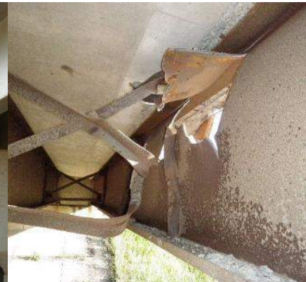
Condition State 4 (Damage)
