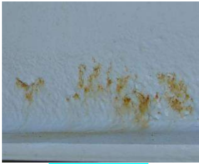
(1000 – Corrosion) Condition State 4
