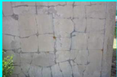
(1130 – Cracking/RC and Other) Condition State 3
