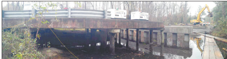
Crews put in new supports as they replace a bridge on Old Bluff Road in Richland County.
