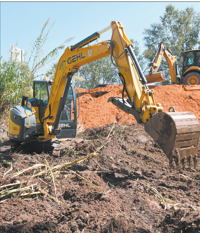
SEPT. 20: SCDOT Florence Maintenance backhoe operators Danny Bostic, background, and Devell Eaddy work to repair a shoulder failure off U.S. 1 in Marlboro County.
