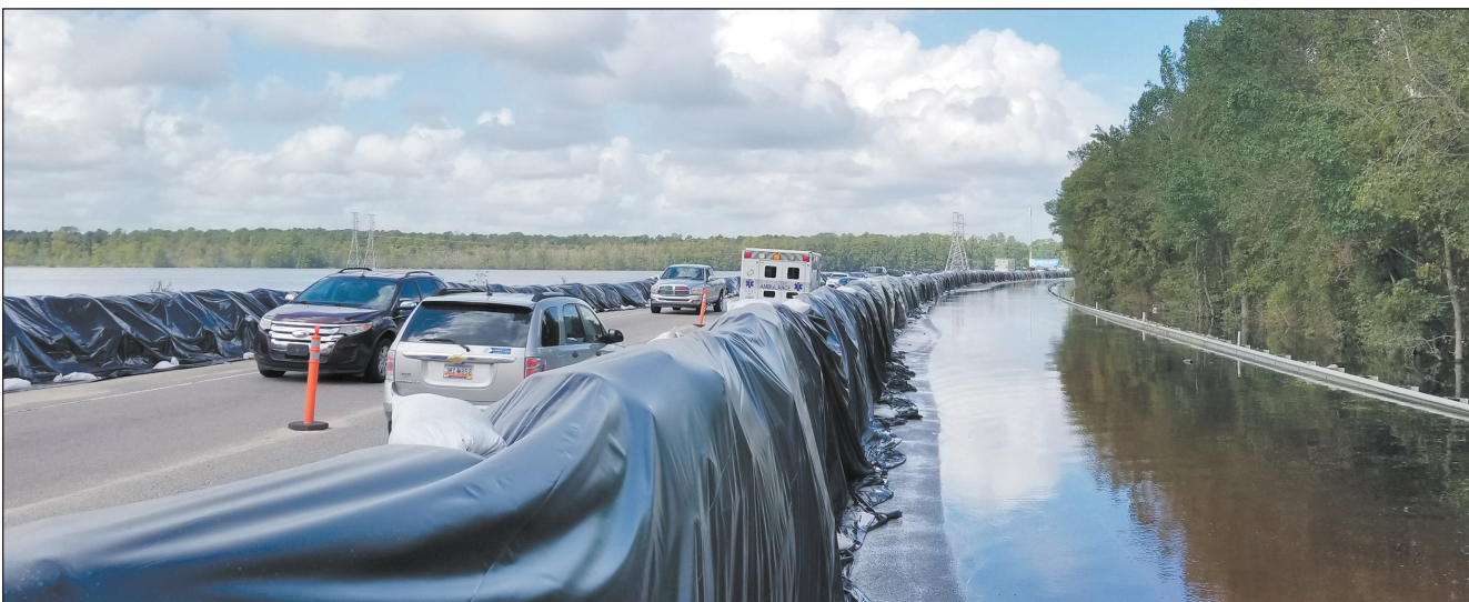
SEPT. 25: Water eventually rises to touch the flood barrier wall. Two lanes of traffic were able to remain open due to the Project Lifeline effort.
