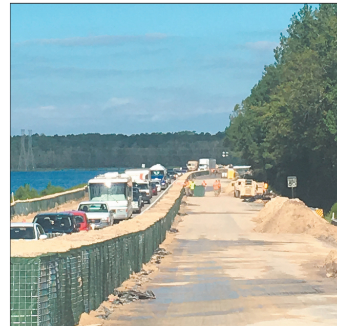
The HESCO flood barrier in Conway was built to keep U.S. 501 Bypass passable when floodwaters made their way down river after the storm.
