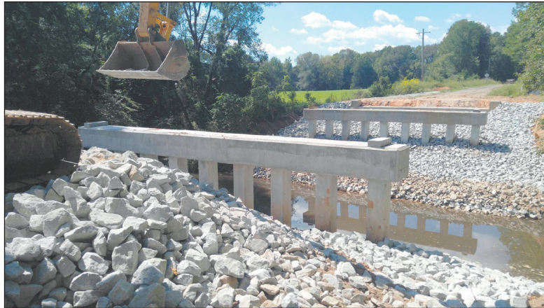
SCDOT's D1 Bridge Crew installs new bridge supports on the Wildflower Road bridge in Richland County.
