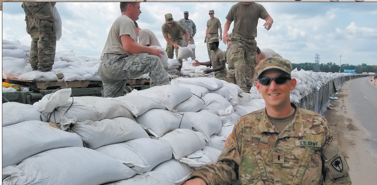
SEPT. 21: SCDOT Saluda Assistant Construction Engineer Garrett Dorn works with fellow National Guardsmen as they make final barrier wall preparations along the U.S. 501 Bypass before expecting flooding from Hurricane Florence.
