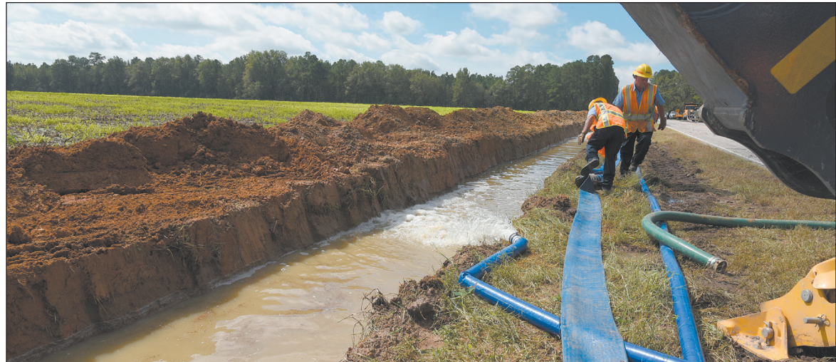
SEPT. 28: SCDOT crew members dig ditches and pump out water to reduce floodwater ponding on Hartsville Highway (U.S. 15) in Darlington County.
