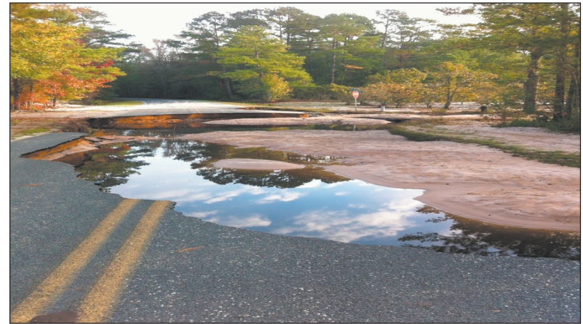
More than 23 inches of rain fell over most of the district. Here is damage to a road near Pee Dee State Park.
