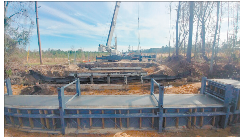
Crews complete the pouring of an end cap on one of the Tram Road bridges in Lee County. In the background, piles are being driven in for the second bridge.
