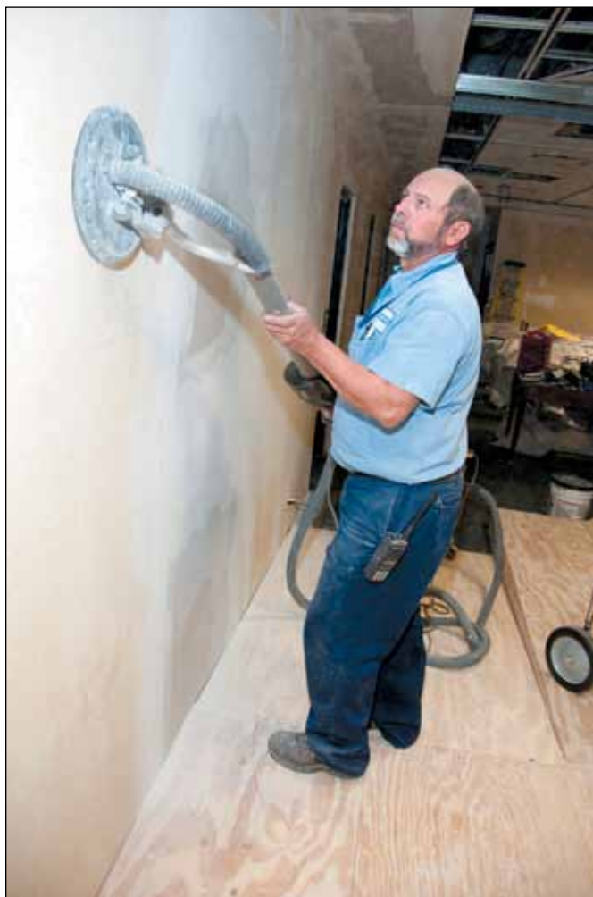
Cal Boland sands the auditorium walls prior to the installation of wallpaper.
