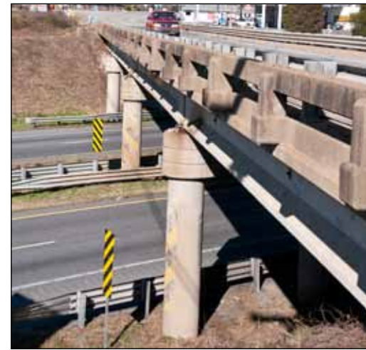
RIGHT: The S.C. 29 Bridge over I-85 in Cherokee County is on the rehab list of projects.
