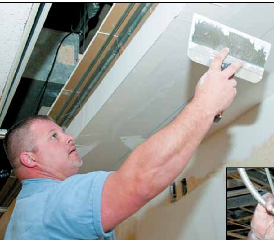
Chris Huepenbecker smooths out the mud while doing sheetrock work along the ceiling of the auditorium.
