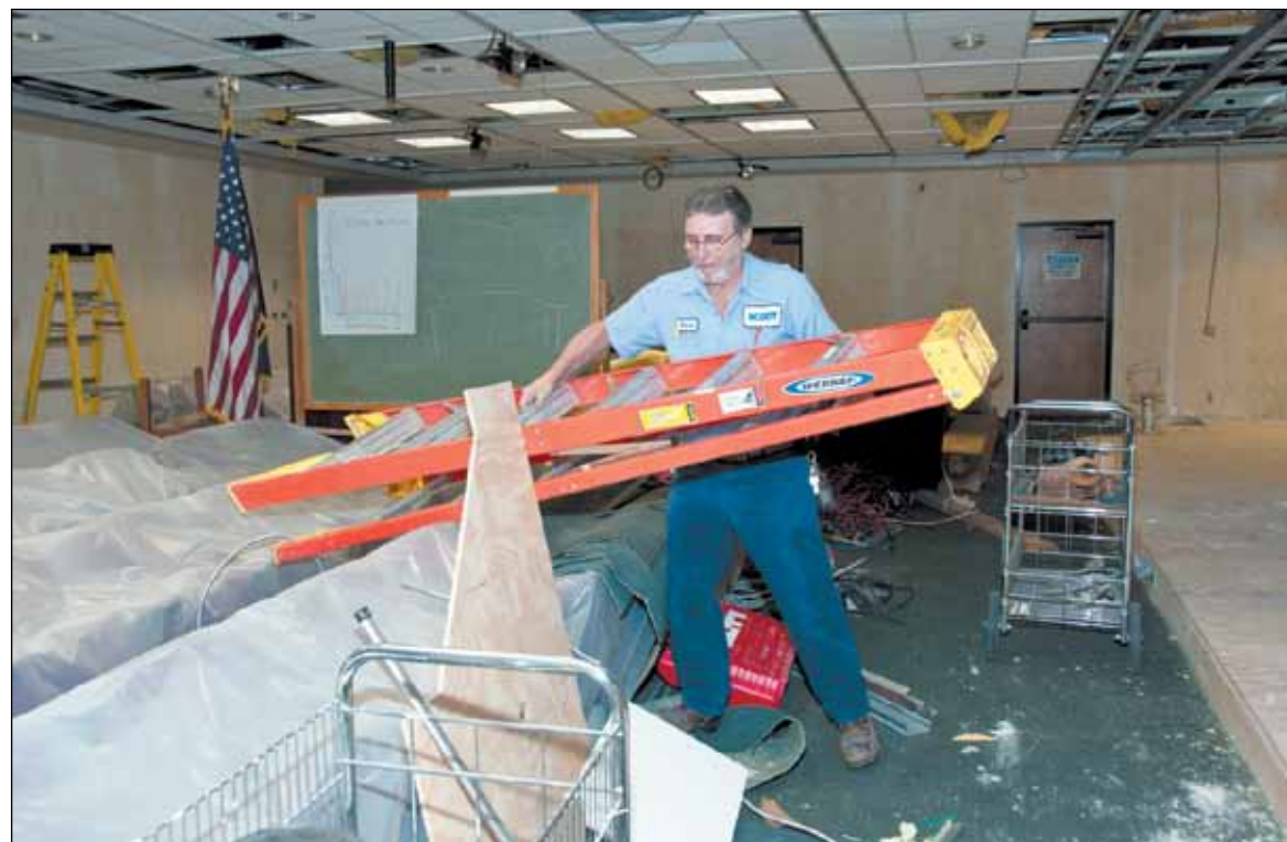
Steve Medlin moves a ladder while working on ceiling tiles, electrical wiring and lighting.
