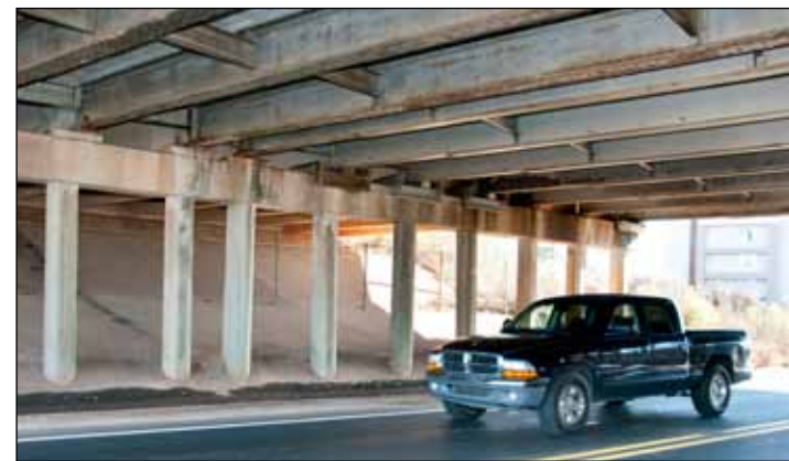
The I-85B bridge over Howard Street (Secondary 2) in Spartanburg will be replaced under the new program.
