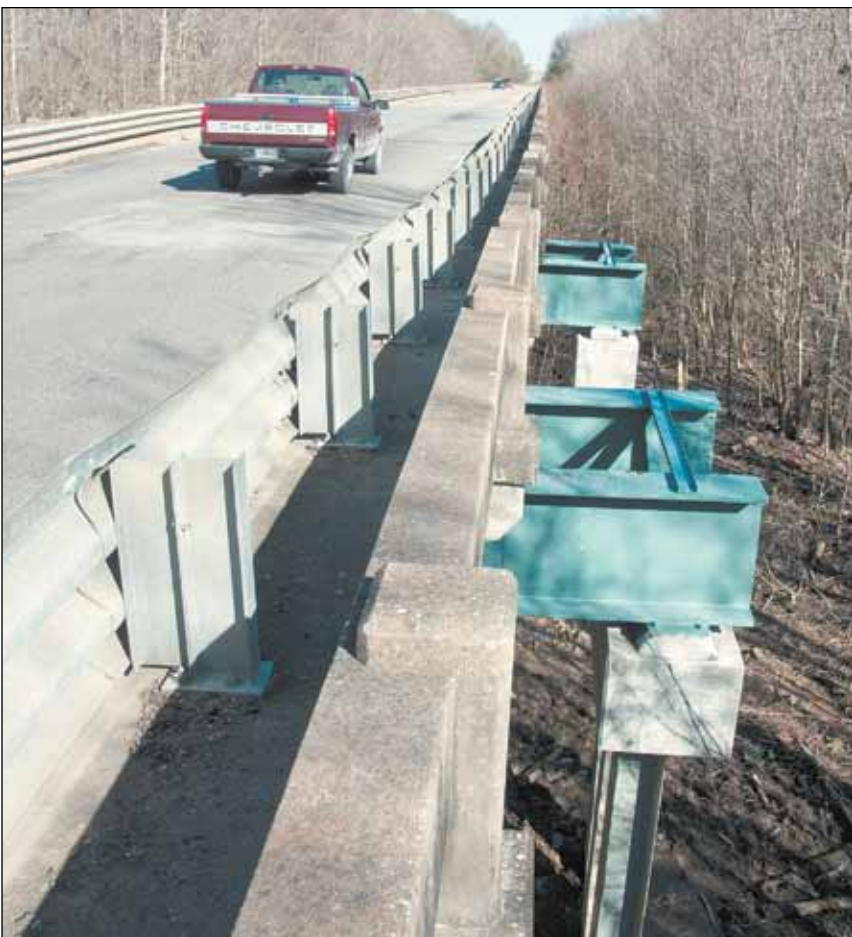
Supports were added to the U.S. 701 bridge over Yauhannah Lake on the Horry/Georgetown county line.
