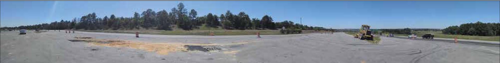
A panoramic view of the crossover point of I-26 at I-77. This is where traffic coming in the eastbound lanes from Charleston will cross back into normal westbound lanes of traffic. It is also the central point of communication for crews in the field during the exercise.
